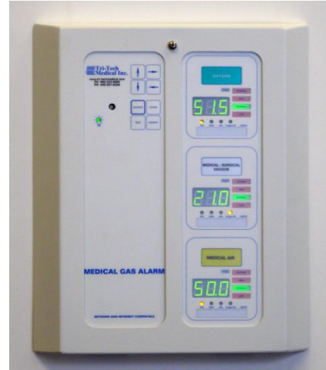
(Area alarm shown is 3 gases – part # DUXXOVA)
